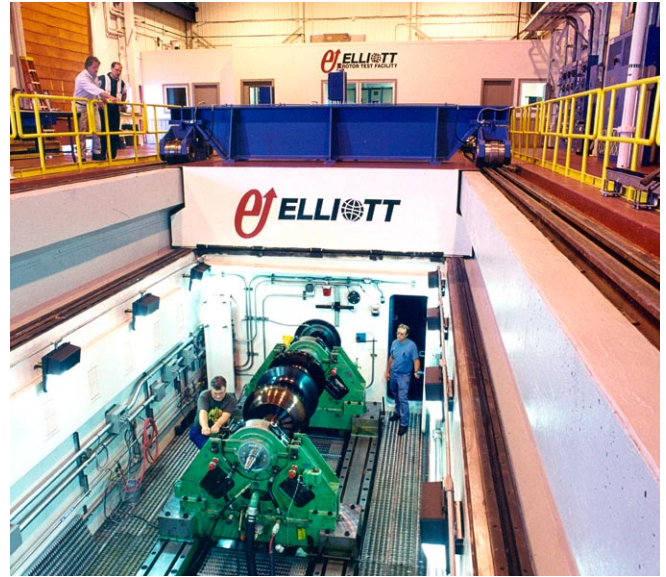
Elliott's state-of-the-art bunker system
